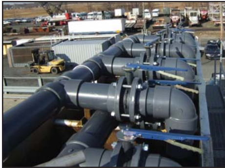
The oil distribution system and recovery tank manifolds were fitted with a six-inch pipes for safe pumping and distribution of oil.
